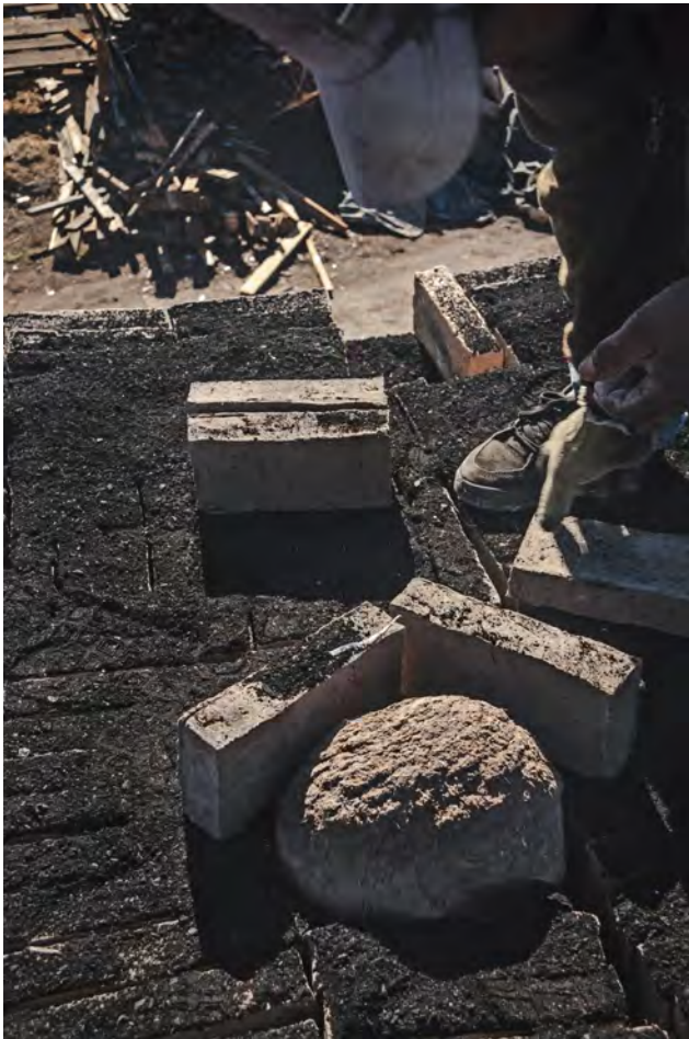
Figure 0.9 Construction of a brick kiln. Each layer of bricks is coated with charcoal, which helps amplify the heat during the firing process. A hornero nest is fired in the oven along with the bricks. Mario Caporali, courtesy the artist
